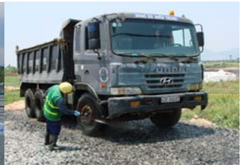
Washing truck tires to prevent contamination from leaving the project site (Photo: TetraTech)
