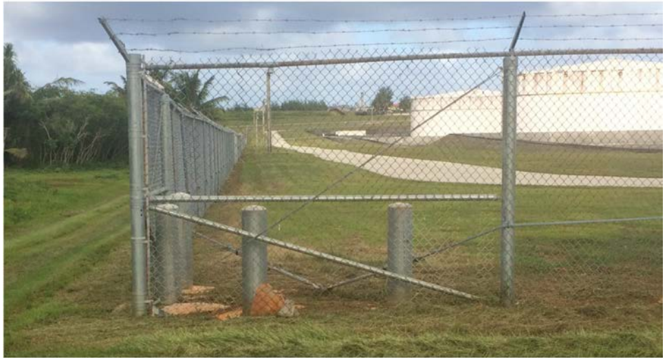
Figure 13: Fenceline Testing Site Near the Fuel Storage Tanks at Andersen Air Force Base, Guam
