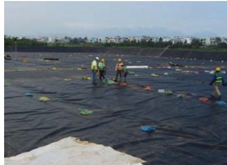
Installing HDPE liner at the bottom of the drying pad (Photo: CDM Smith)
