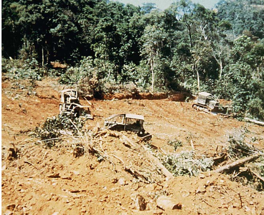
Figure 3.27 A photograph of US Army Corps of Engineers using Rome plows to clear vegetation in III Corps, Vietnam (Photograph courtesy of J. Ray Frank, Frederick, Maryland)
