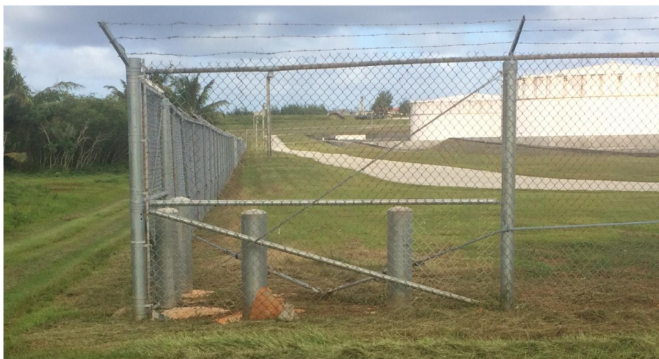
Figure 13: Fenceline Testing Site Near the Fuel Storage Tanks at Andersen Air Force Base, Guam
