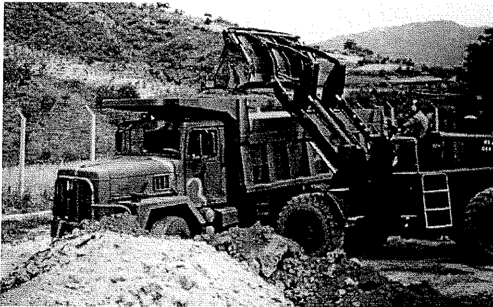
» A photo of heavy machinery mobilized for a landfill operation at Camp Carroll. The landfills were revealed through disclosure from U.S. Army veteran Steve House. (Yonhap News)
