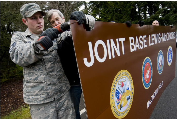
Staff Sgt. Jeffery Cardinal, left, and Craig Hayes, 62nd Civil Engineer Squadron, drill holes in the new Joint Base Lewis-McChord sign at the main gate Sunday in preparation of Initial Operational Capability of Joint Base Lewis-McChord. (U.S. Air Force Photo/ Abner Guzman)
